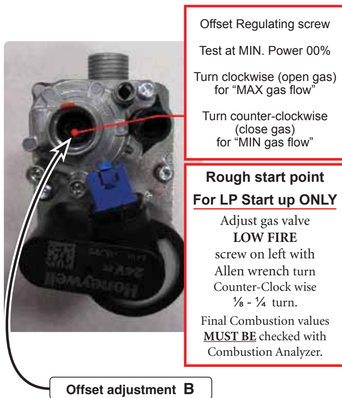
Figure 105 Offset adjustment screw — (ONLY for use by a qualified technician, using calibrated combustion test instruments).
