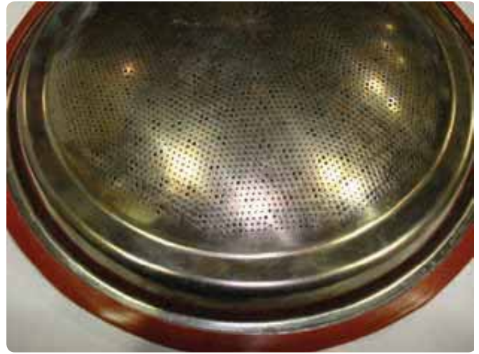
Figure 144 Inspecting exterior and cleaning the burner
